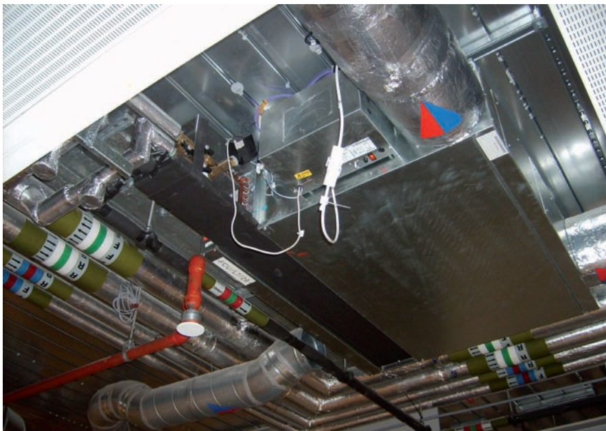
An installed fan coil
