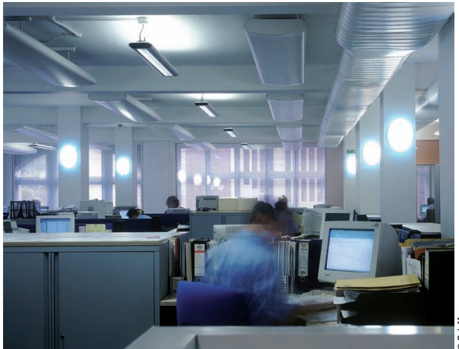
Chilled beams within an office space
